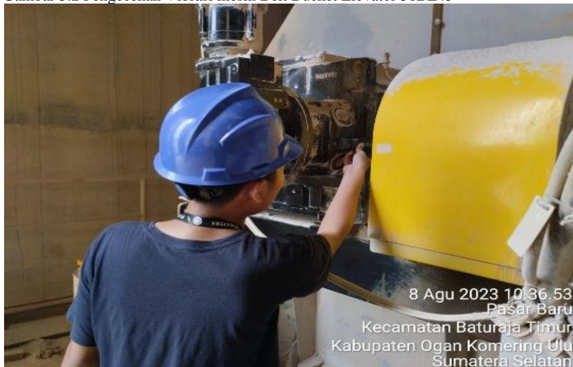
Gambar 3.2 Pengecekan Vibrasi mesin Belt Bucket Elevator 51BE45
