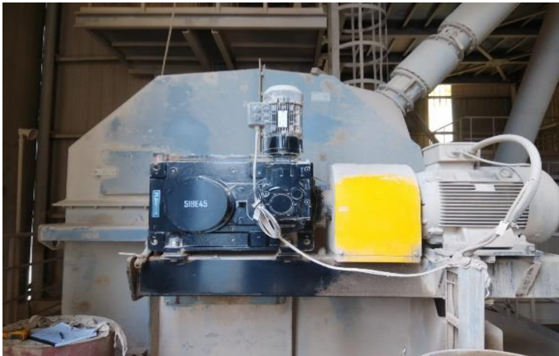
Gambar 3.1 Mesin Belt Bucket Elevator 51BE45
